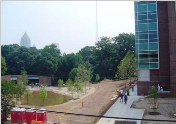
The Molecular Science and Technology building is receiving its final touches. It will be ready in October 2006.
