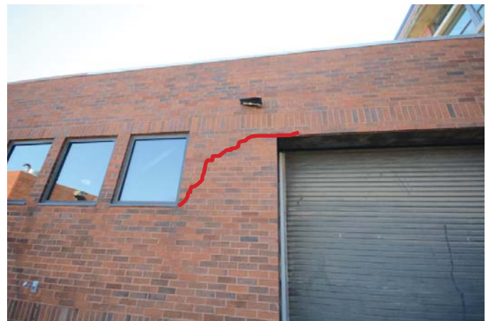
Figure 33: A large crack in the veneer (center) extends from the window sill to the corner of the overhead door opening.
