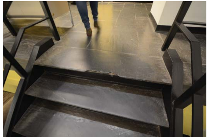
Figure 32: Chipped nosing on the slate treads in New Rich.
