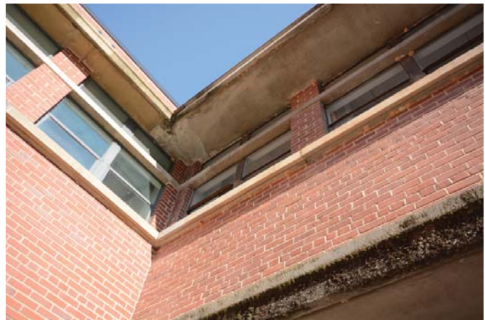
Figure 25: Stains and insect nests are visible on the exterior surfaces of the Calculator Building.
