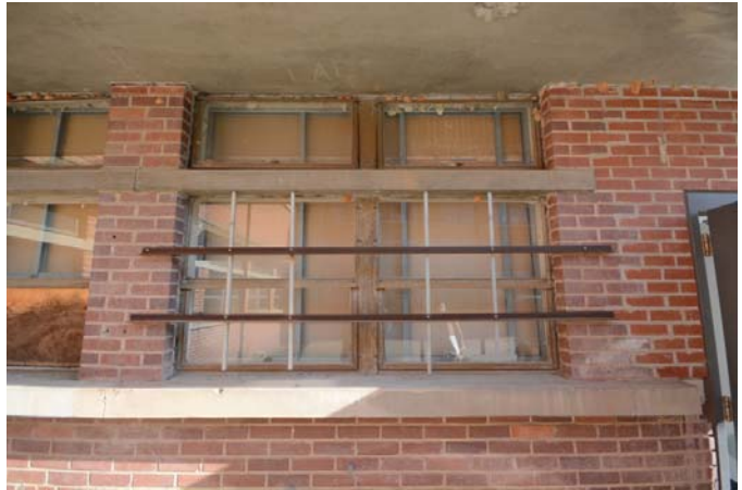
Figure 13: Calculator Building ground floor windows, south elevation, boarded up from the interior.
