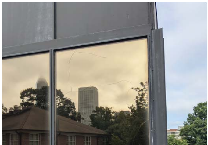
Figure 30: Penthouse windows showing fogging (condensation) and cracks.
