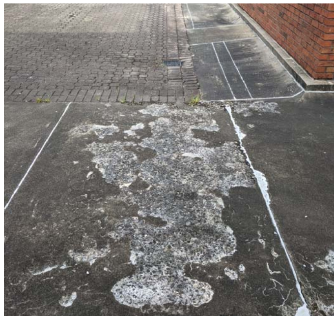
Figure 28: 1971 Rich building roof showing spalling concrete and sealant in joints.
