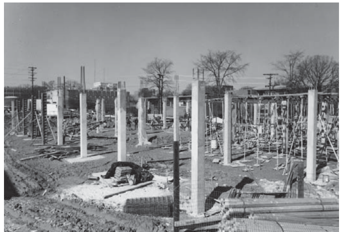
Figure 19: New Rich under construction, c. 1971. Georgia Tech Library, Archives and Special Collections.
