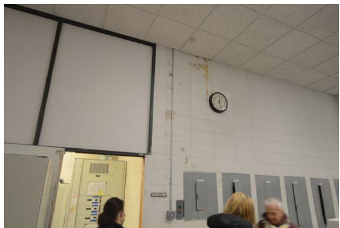
Figure 31: Water stains are visible on the wall (center) in one of the server rooms.
