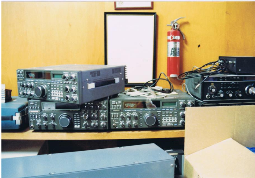
Figure 7-3 - Buz Reeves' shack is packed for shipment to W 4 AQL. Here are three of the Kenwood TS-940S HF radios used at K 2 GL. The club kept two but sold the rest. To the right is an older Drake TR-7 transceiver that was used before the Kenwood radios were purchased.
