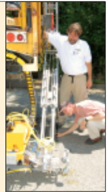
ABOVE: During a June 2006 demonstration, GTRI researchers Wiley Holcombe, standing, and Steve Robertson examine the placement mechanism on truck-mounted, automated raised pavement marker (RPM) placement machine that GTRI developed for the Georgia Department of Transportation.
