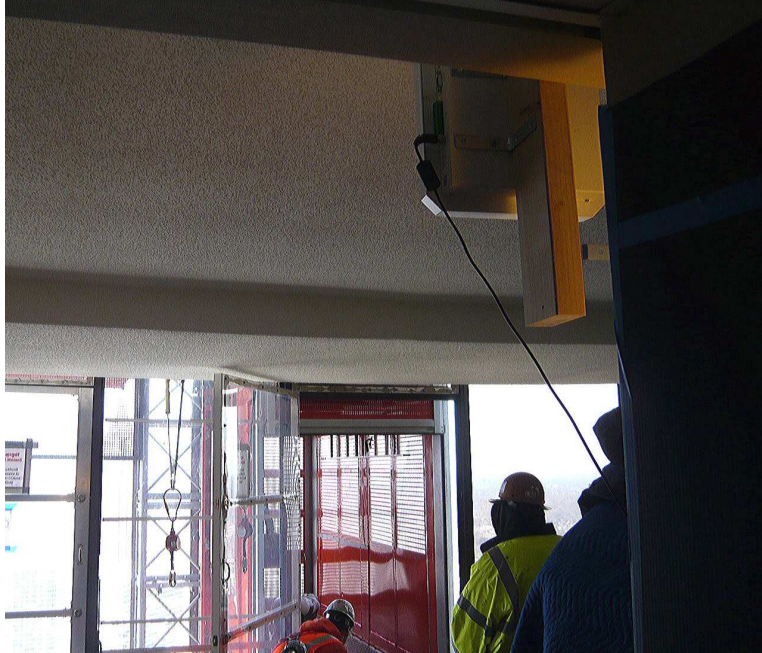
Figure 4.6 Reader Installed Across from Material Hoist on Floor 63
