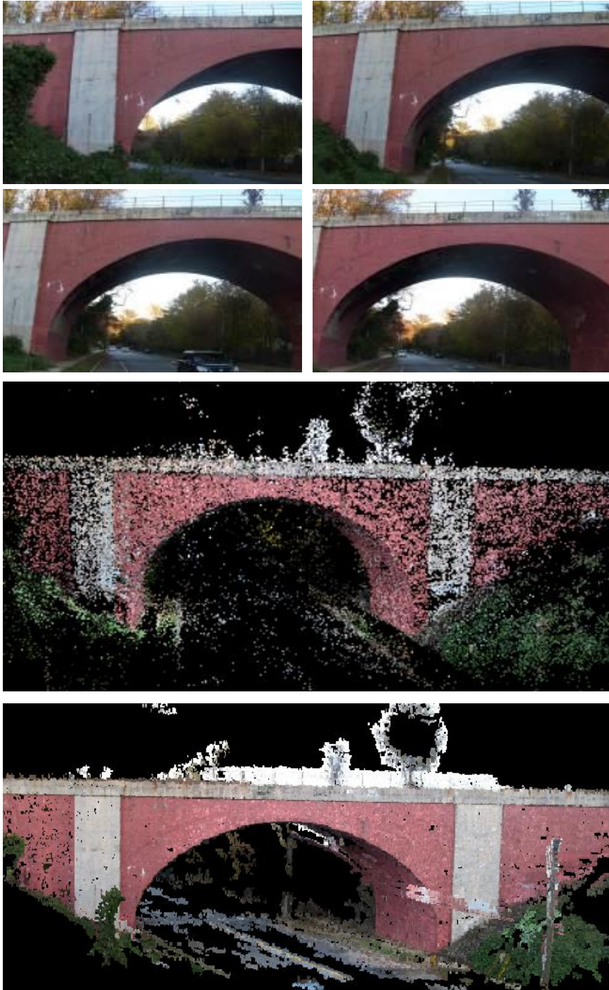
Figure 5.9: Outdoor case study #02: concrete arch bridge: point cloud data before improvement (middle) and after improvement (bottom)
