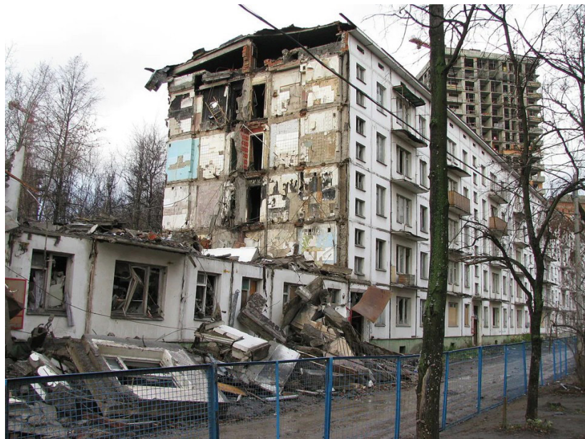
Figure 1: Half-demolished panel-constructed residential building with a new development under construction in the background, Moscow. Source: Archinect 2017.
