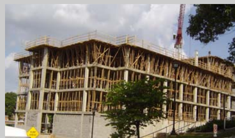
Molecular Science and Engineering Building Due to open in the Fall of 2006.
