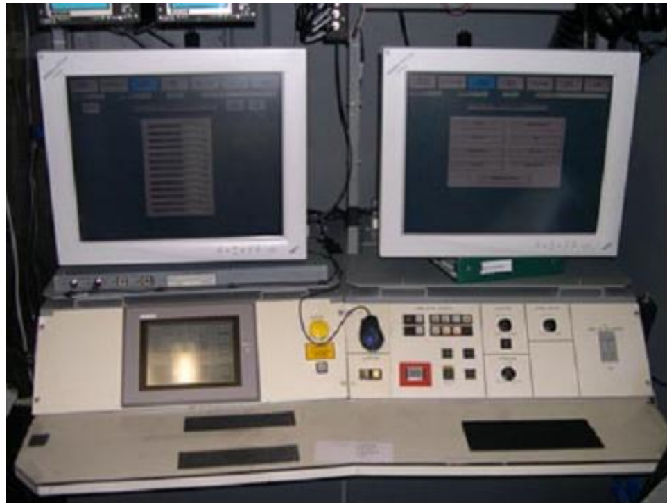
Figure 5.2: NUH-60 Observer/Operator Console
