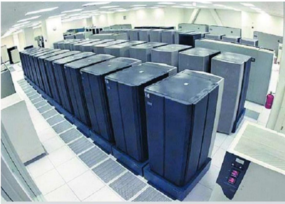
Figure 1.1. A typical data center [1]
