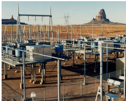
Figure 2.13: Image of 230 kV, 330 MVAR TCSC at Kayenta, U.S. (Courtesy: ABB).
