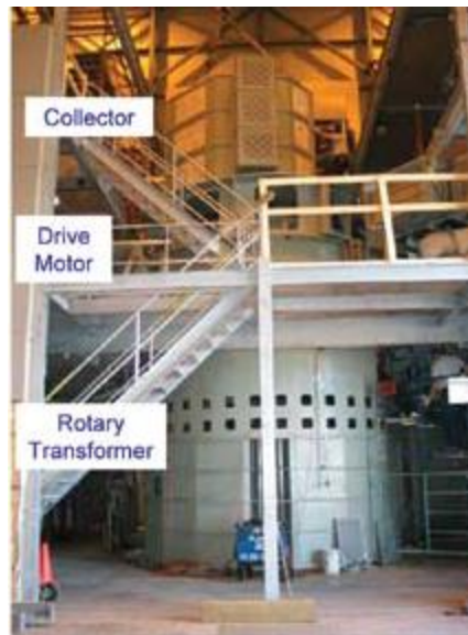
Figure 2.17: Image of 100 MW VFT at Langlois, Canada-USA. (Courtesy: GE)
