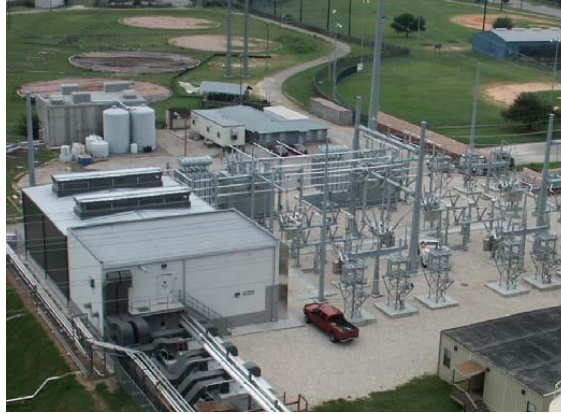
Figure 2.7: 138 kV, +/- 95 MVAR STATCOM at Holly substation, U.S. (Courtesy: ABB)
