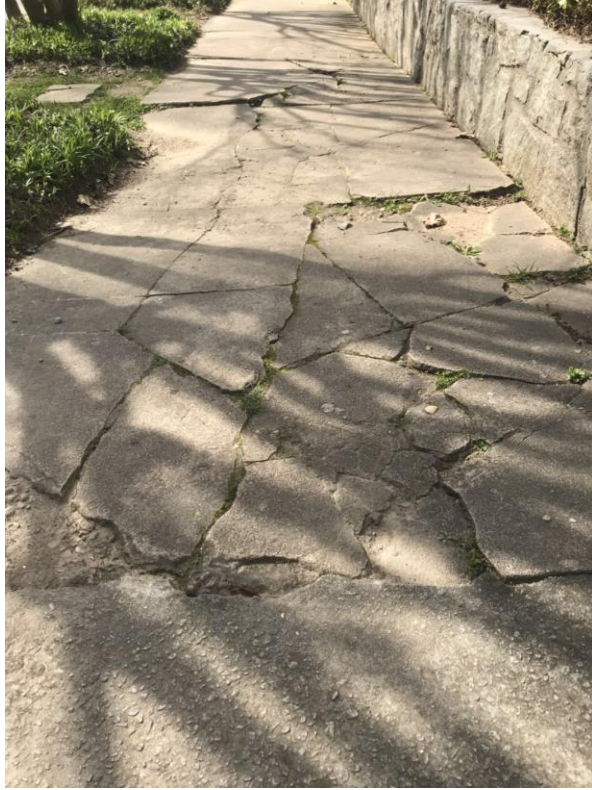
Figure 6. The Surface Crack along the Control Route.
