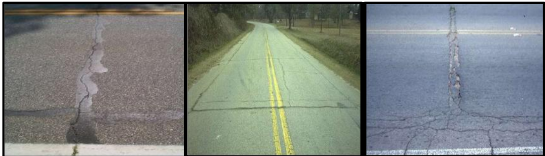
Figure 4: Illustration of severity levels of reflection cracking (Level 1 to Level 3)
